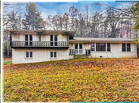
NORTH CAROLINA WATER DAMAGE
